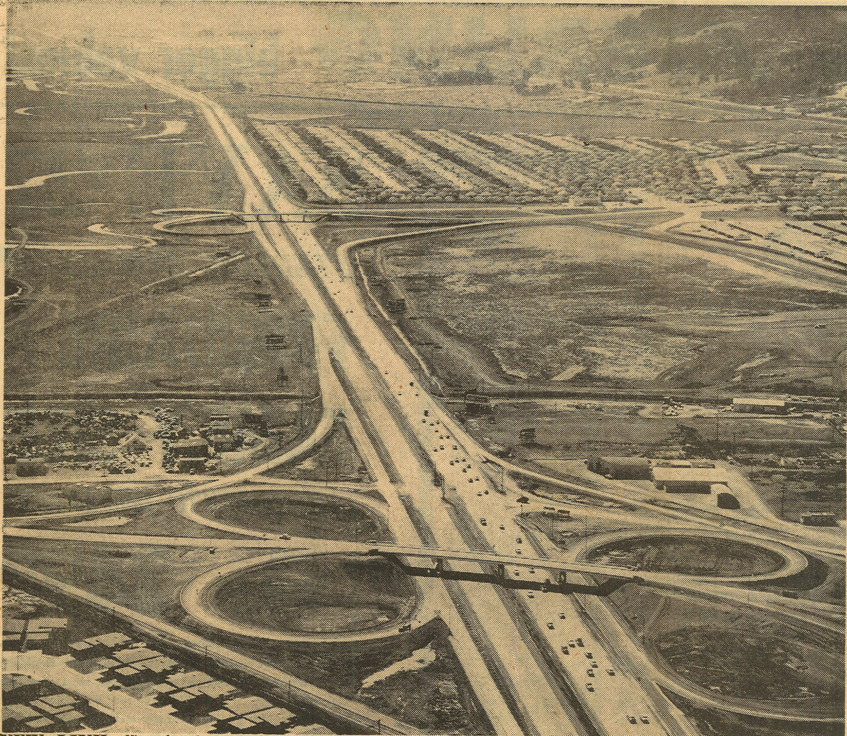
NEW LINK —View of newly completed northbound lane of the Bayshore Freeway between San Mateo and San Carlos. Although this work is completed, motorists are urged to use caution as construction still is under way on four interchanges. Shown in foreground is one at Nineteenth Avenue and just beyond is the one at Hillsdale. The other two are beyond at Belmont and San Carlos.
